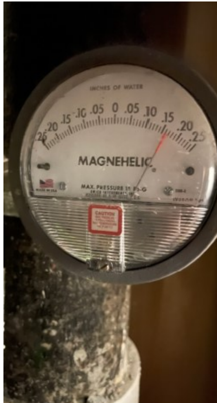
Photo 3 - View of Riser 4 gauge.
