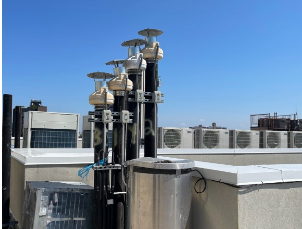
Photo 6 - View of riser exhausts on roof.
