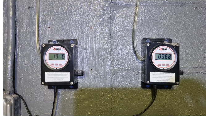
2. Typical audible alarms, suction points RP-1 and RP-2
