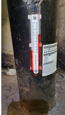
1. Typical U-manometer reading, suction point SP-1
