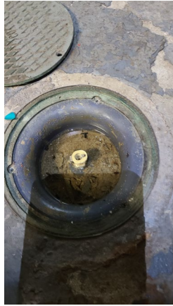
5. Excessive water at SSMP VM-06
