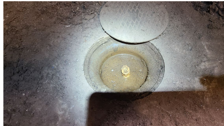
4. Excessive water at SSMP VM-01
