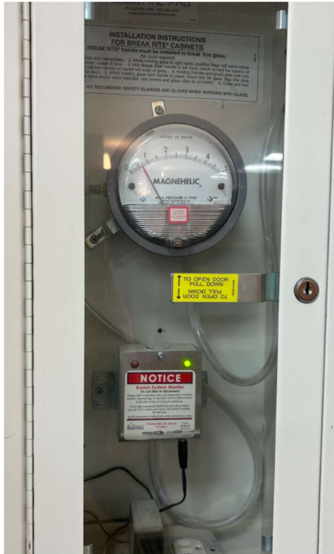
Photo 5: Alarm / Magnehelic for Fan 3
