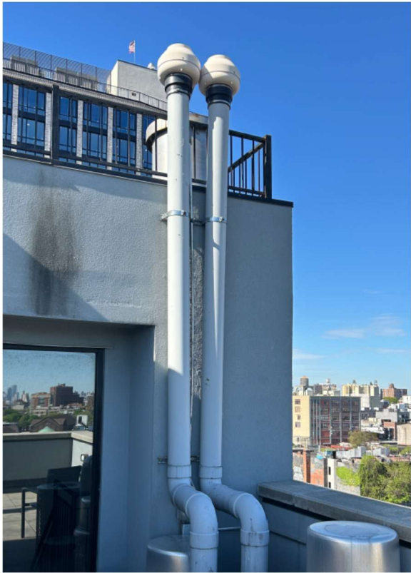
Photo 1: Risers and Fans for Loop 1 and Loop 2
