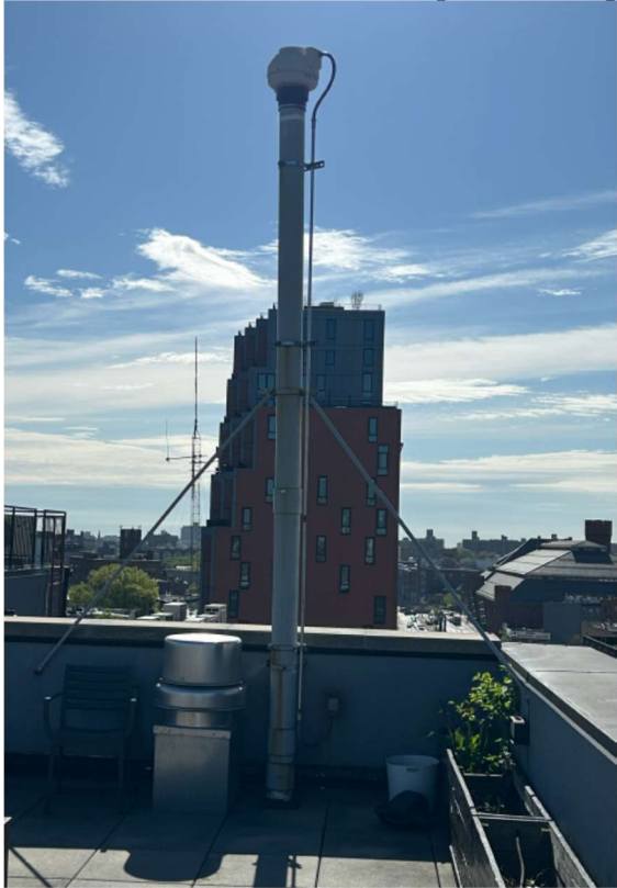
Photo 2: Riser and Fan for Loop 3
