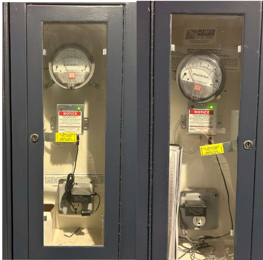
Photos 3 and 4: Alarms / Mangelic Gauges for Fan 1 and Fan 2
