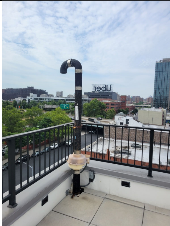
SSDS Vent on the Roof
