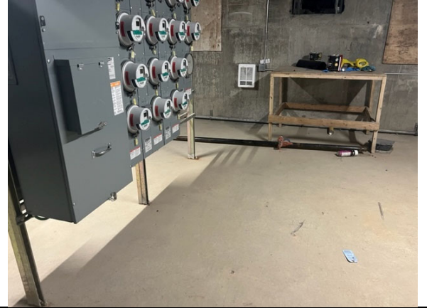
Basement Floor and Electrical Meters
