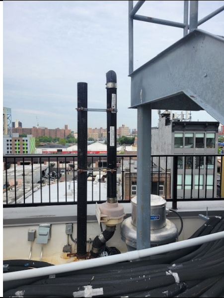
SSDS Vent on the Roof
