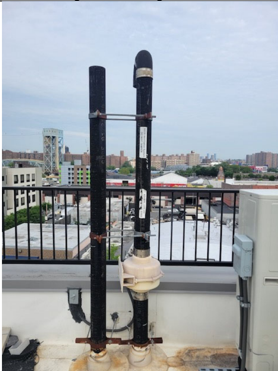
SSDS Vent on the Roof
