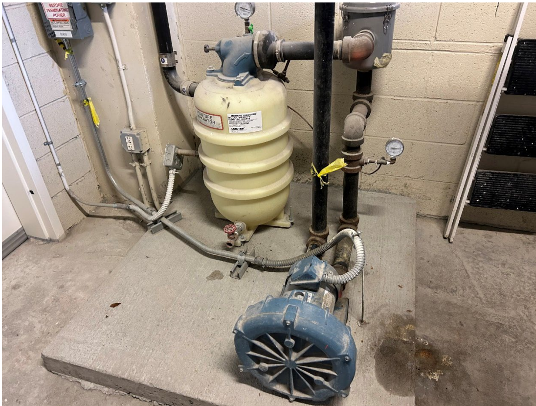
Photograph 8: View of SSDS blower.
