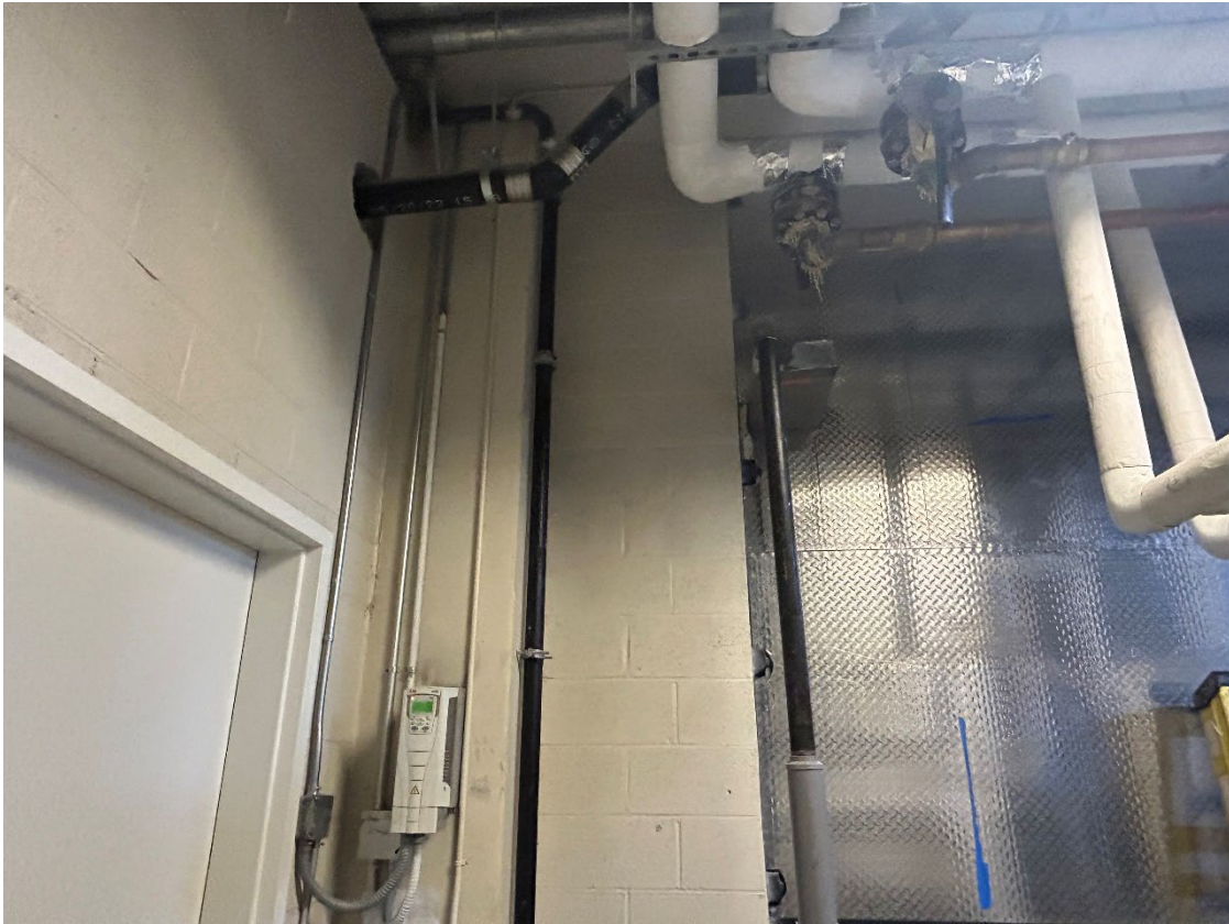
Photograph 11: View of SSDS piping from blower through the wall.
