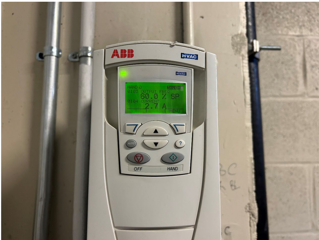
Photograph 12: View of the VFD for the system.
