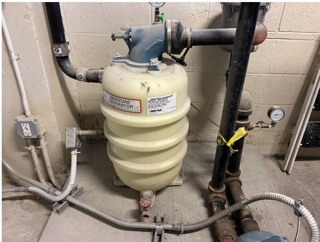
Photograph 6: View of knockout tank for the SSDS.
