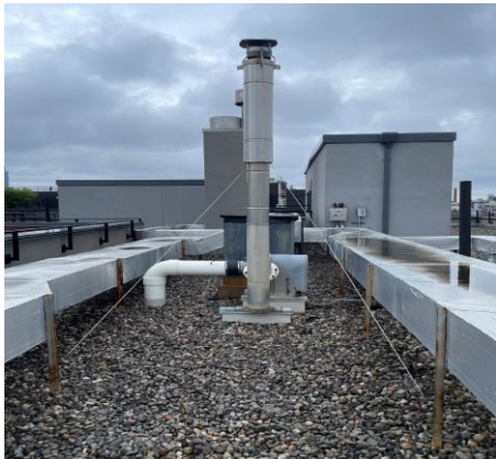
Photograph 2: Exhaust stack on the roof.
