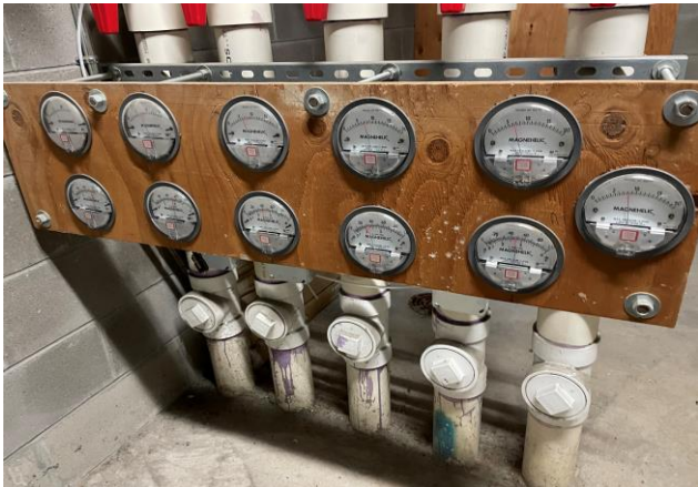
Photograph 1: SSDS Air Flow and Vacuum gauges.
