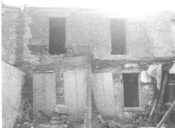
23. View of the fire-damaged portion of the subject property building and vacant building to the west (facing south).
