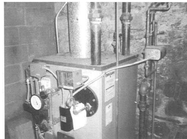
18. View of boiler in eastern basement.
