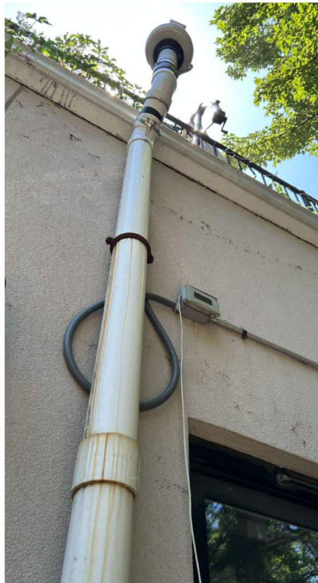
Photo 2 – View of riser included. Due to access issues, couldn't get a photo of the blower at the roof. However, vacuum was observed within the magnehelic and the blower was operable.
