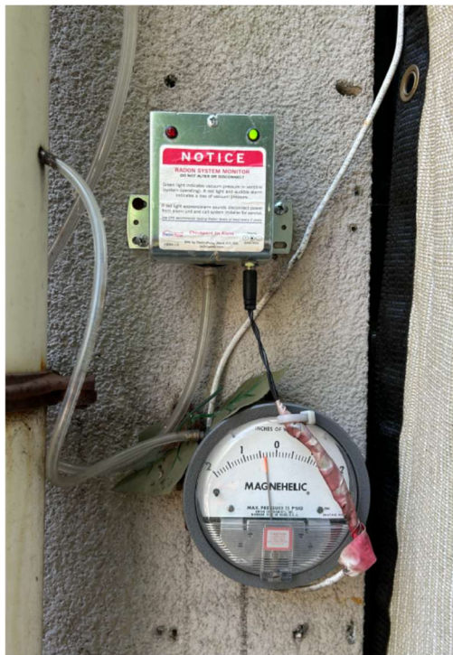
Photo 1: View of alarm and magnehelic
