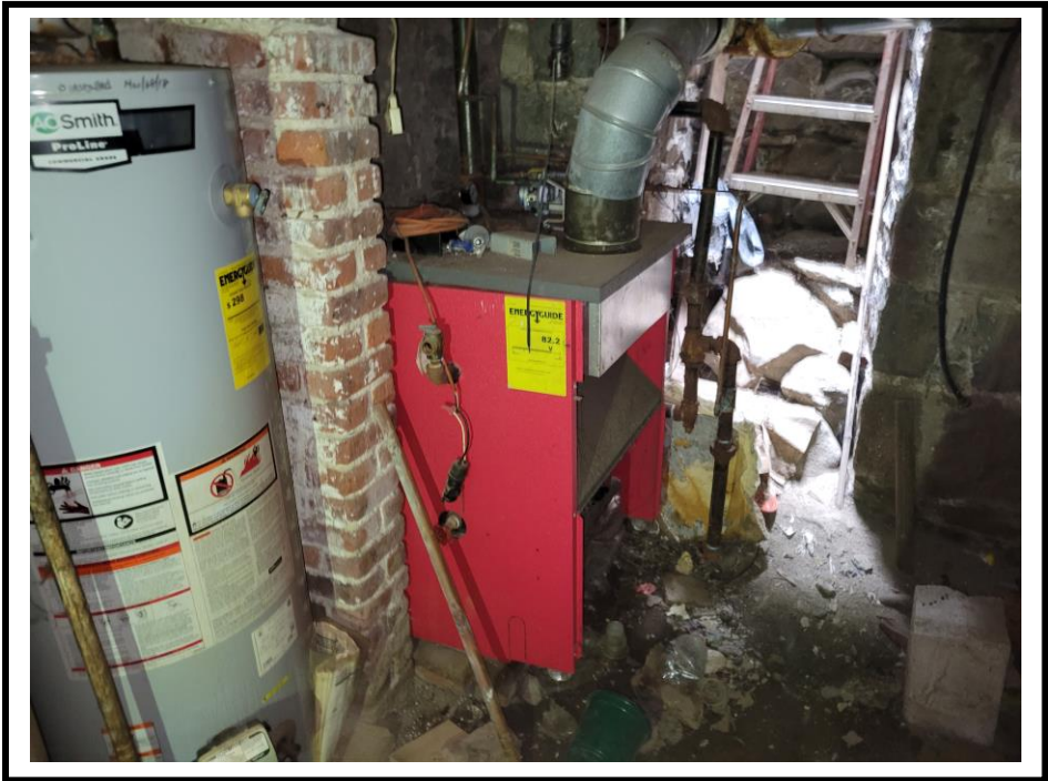
PHOTO LOCATION: Depicts one of the two water heating tanks and the boiler in the cellar.
