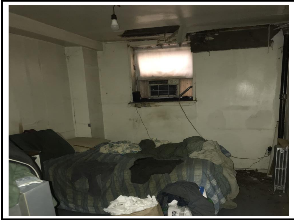
PHOTO LOCATION: Depicts the bedroom in the rear apartment unit on the first floor, with damage on the ceiling.
