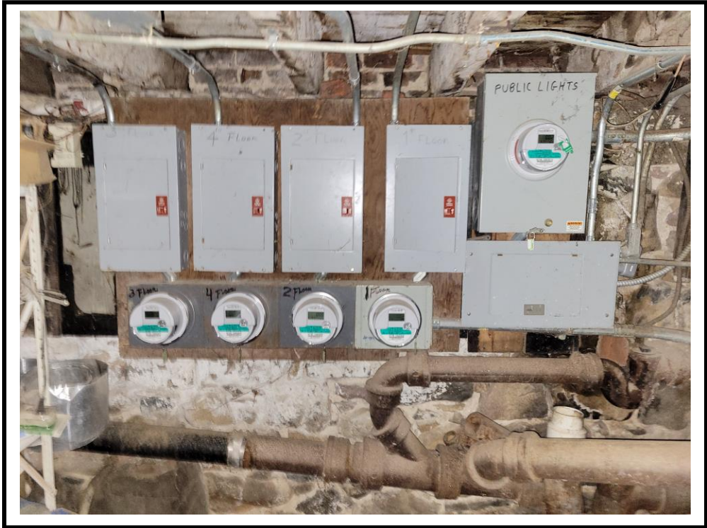
PHOTO LOCATION: Depicts the electrical meters for the residential units in the cellar.
