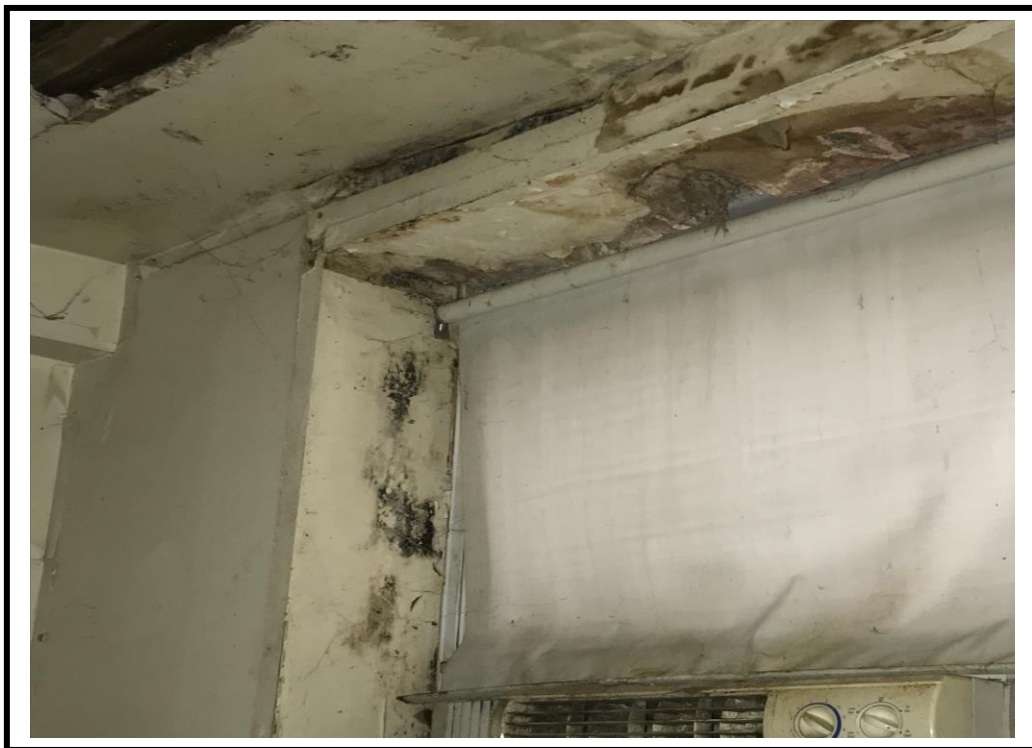
PHOTO LOCATION: Depicts water staining damage with black mold on the interior window frame in the bedroom.
