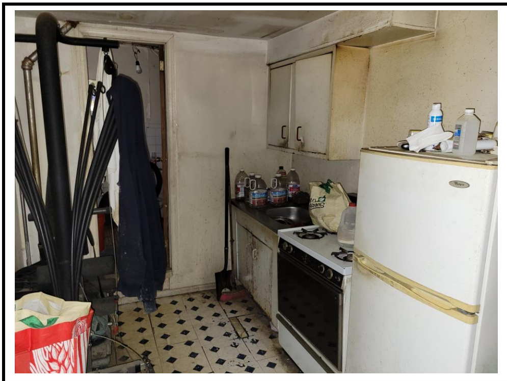
PHOTO LOCATION: Depicts the kitchen in the rear apartment unit on the first floor.
