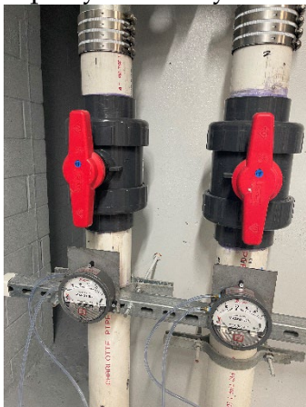
SSDS Manifold Piping and Pressure Gauges
