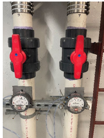
SSDS Manifold Piping and Pressure Gauges
