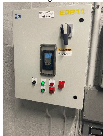
SSDS Power Panel
