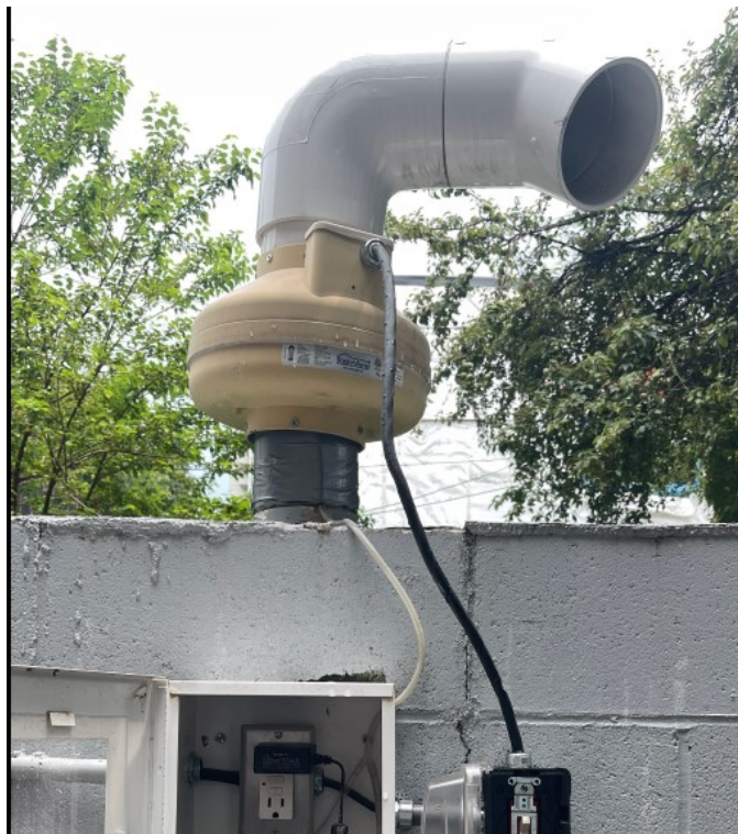
Photo 2: View of the riser above the fan in the rear parking area of the Site.
